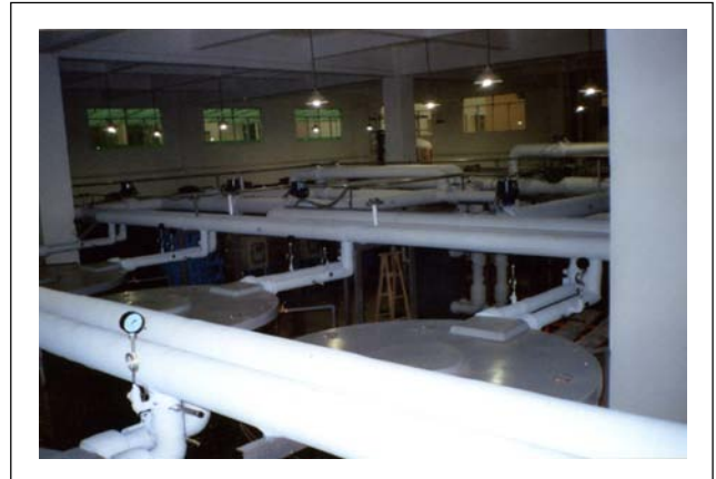
儲冰槽現場配置與配管 Local layout and piping of ice storage tanks
